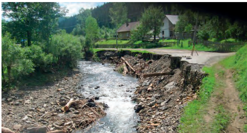
Fig. 10.1.2. Road in Lopushne village, destroyed by the lateral erosion
